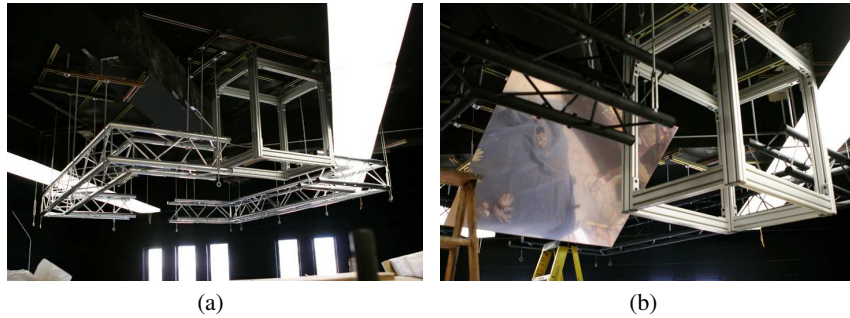
Fig. 4. (a) Screen hanging cables, aluminum trusses mounted to the ceiling, and (b) aluminum trusses painted in black to minimize light reflection and the floor projection mirror
