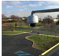
Figure 12: PTZ camera installed on the roof for data collection.
